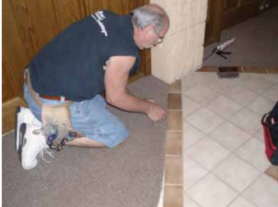
Professional carpet installer Dave Pethan carefully peels back the carpeting under which the hearing loop will run.
